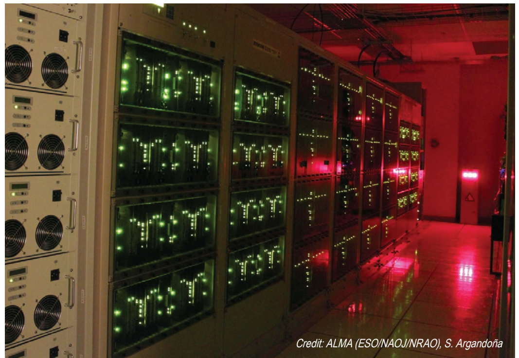
Fig. 4. Image of all 8 racks in one quadrant of the main array correlator in the correlator room at AOS Technical Building. It shows 2 first station racks (with green lights) followed by 4 correlator racks (with green lights and red light reflection) and, at the bottom of the room, 2 other station racks (with green lights and red light reflection). The full system includes 4 identical quadrants for a total of 32 main racks. All racks, adding the power and computer racks, dissipate around 130 kW.
